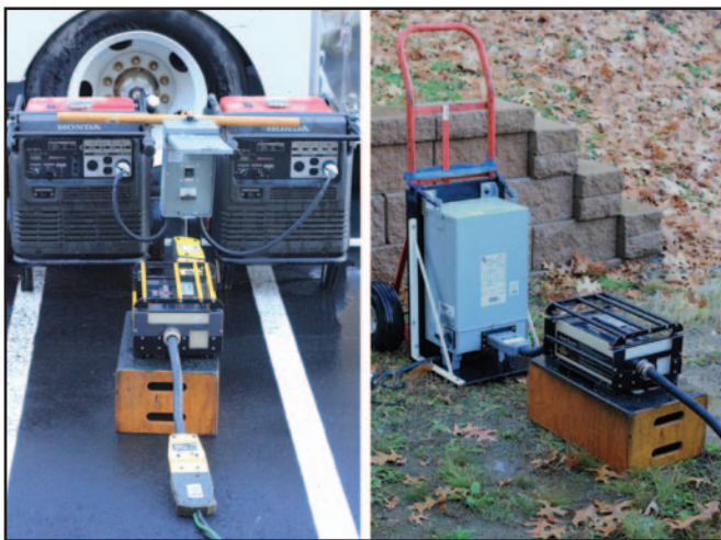
Figure 5 – A tiered strategy for ground-fault protection. A 100 A/240 V Shock Block GFCI (left) provides blanket protection to the 240 V distribution system. A 100 A/120 V Shock Block GFCI (right) provides blanket protection to the 120 V distribution system derived from the 240 V output of the generators by a step-down transformer.
